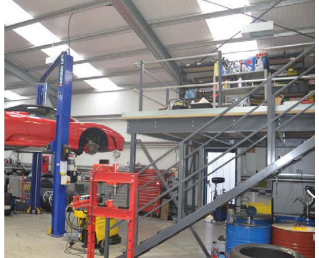
The new mezzanine floor providing a live load of 4.8kN per sq metre and up to 500kg point loading is completed – less than 8 hours after the first photo was taken.
