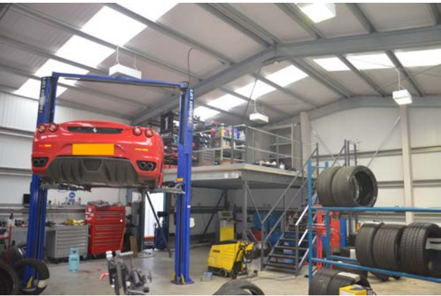
The new mezzanine floor has its shelving installed and parts laid out for storage
