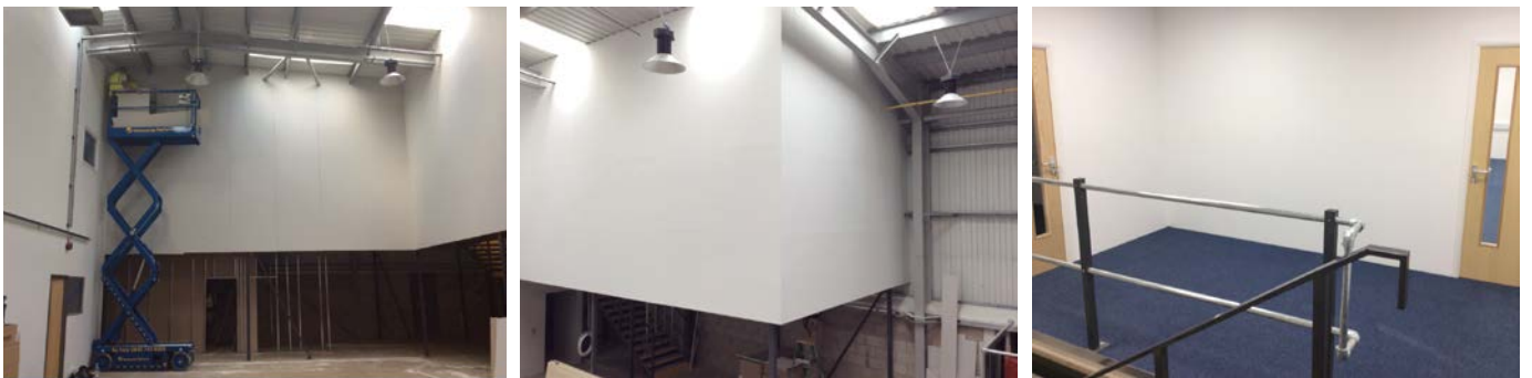
Partitioning is up on the mezzanine. Walls are drylined and painted and carpeting put down.
