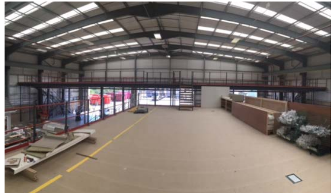
After: View of the industrial mezzanine installed at Prestige and Homeseeker Park and Leisure Homes Rushden by Cubex Contracts
