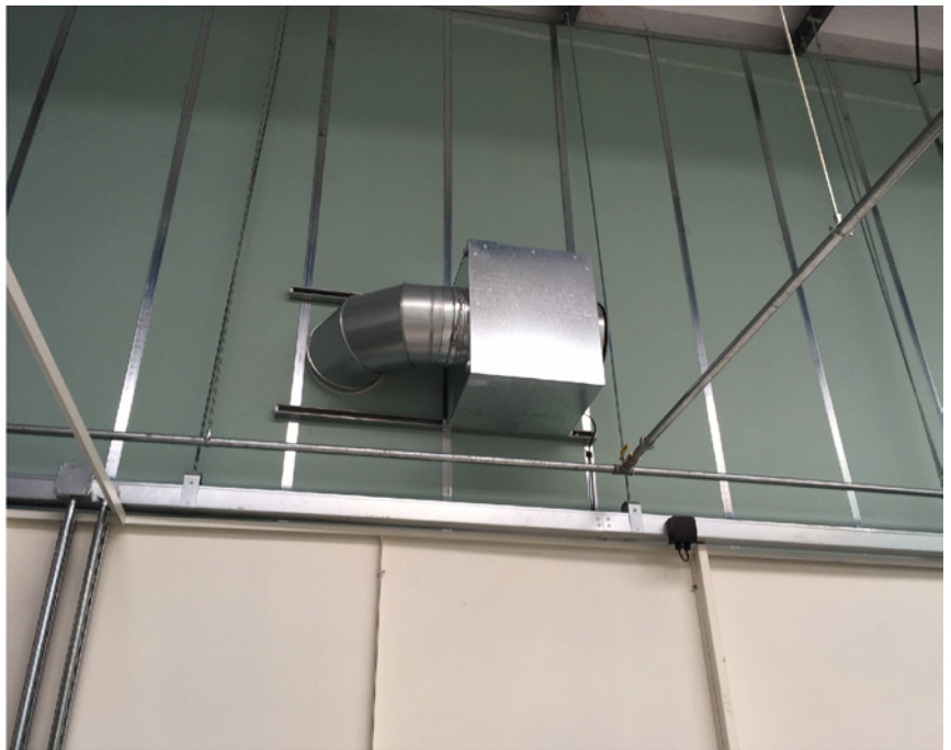
Close up of the extractor fan needed to create clean air flow in the now closed in workshop area.
