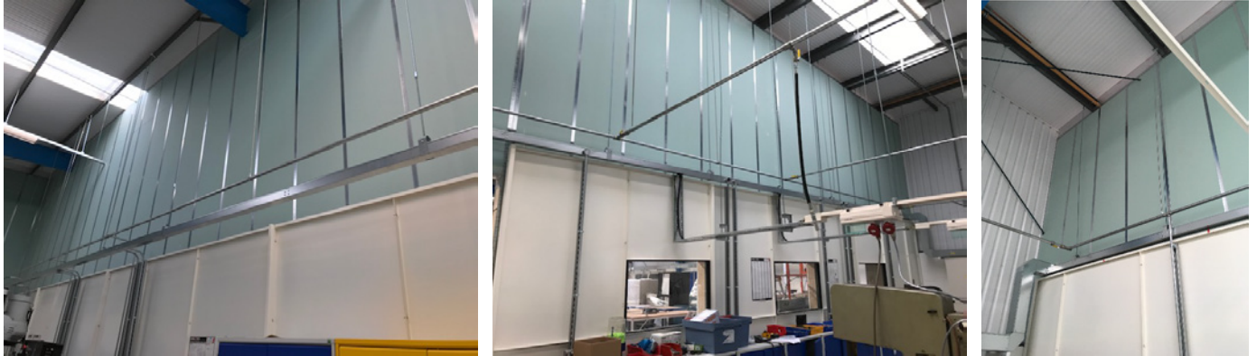
Photos showing the inside of the workshop area where you can see the existing steel partitioning creating the original shell - and now being supported with the shaftwall reaching up to the ceiling to seal the once open space.
