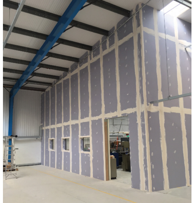
Shaftwall is erected to reach the high ceilings (up to 7m in places), around the existing workshop area.
