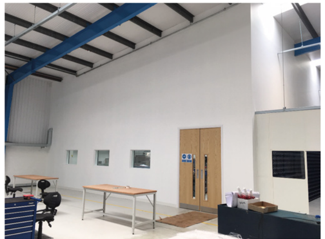
View of the shaftwall after decorating - with acoustic sealed double door and triple glazed windows.
